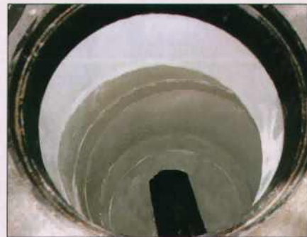
In corrosive environments, a manhole can be replaced without digging by installing a plastic liner fitted to a form, and filling the annulus space between the form and the old wall with concrete.
