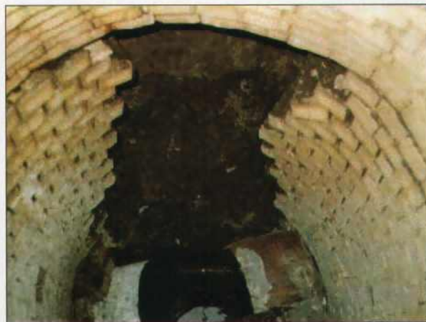
On a brick manhole, water movement can remove mortar, leading to the loss of bricks and eventual structural failure.
