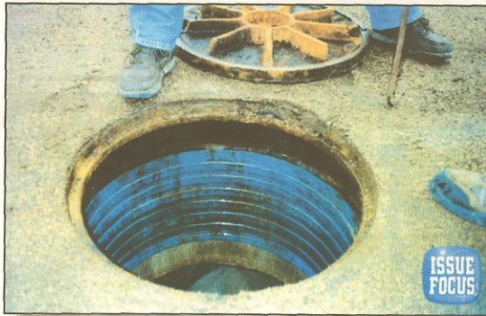
Down the chimney. Close-up of a repaired manhole with a chimney composed of several Ladtech® rings. Ladtech photo
